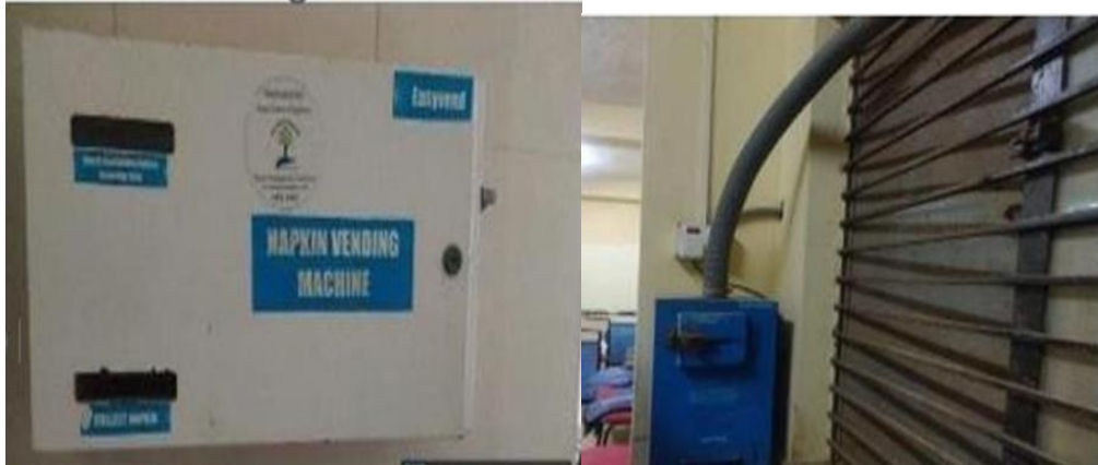
Fig 18: Sanitary Pad Dispenser and Vending Machine
