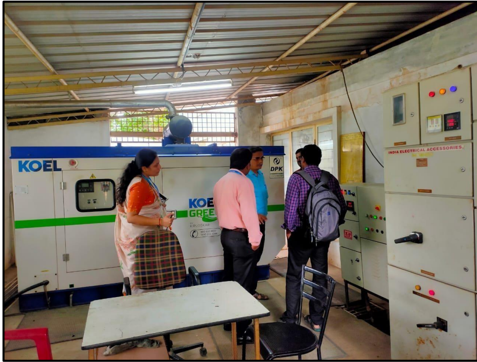
Fig 2: Audit team Visited generator room
